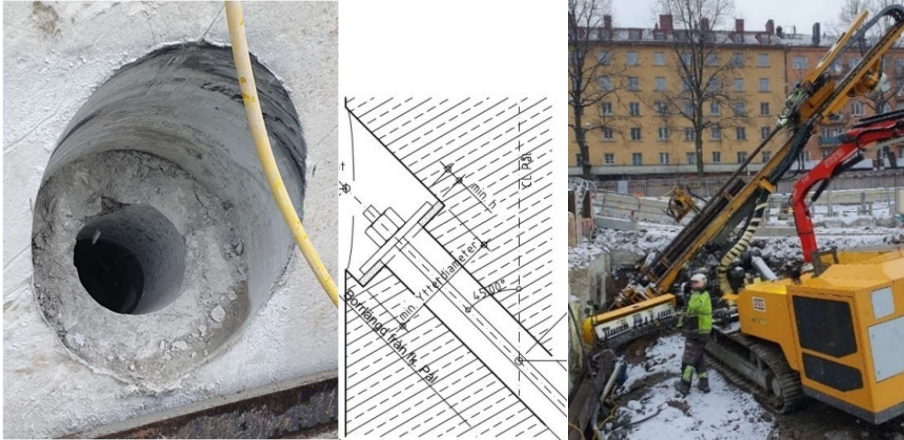
Figure 12 Left and middle– holing in each secondary pile for further anchoring. Right- ongoing drilling for anchoring.
