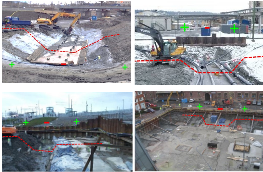
Figure 1. Some typical situations where 3D-effects have been incorporated in design in order to achieve satisfying stability conditions in temporary excavations. Upper left: A battered excavation with a limited horizontal extent. Upper right: A cantilever sheet pile wall next to trafficked railway tracks. Lower left: A cantilever sheet pile wall supporting an excavation that progresses sequentially from right to left while simultaneously casting a concrete slab. Lower right: A sheet pile wall supported by struts while excavating and casting a concrete slab sequentially.
