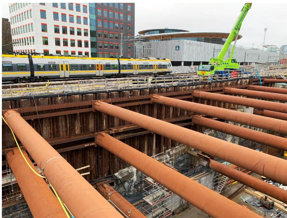
Figure 1: Live railway next to the strut supported deep excavation for the Västlänken-tunnel.
